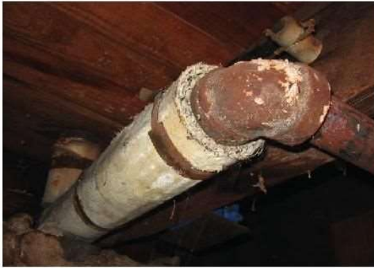
Damaged asbestos lagging
