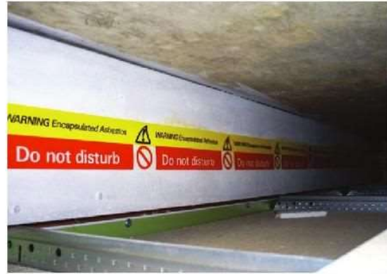
Labelled encapsulated asbestos
