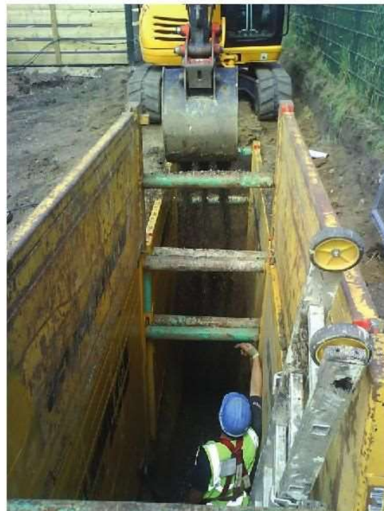
Safe working in a deep excavation using trench boxes and a tied ladder
