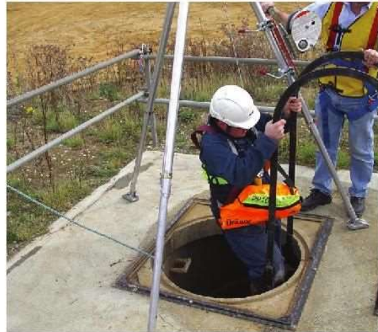
Entry to confined space with lifeline and rescue equipment
