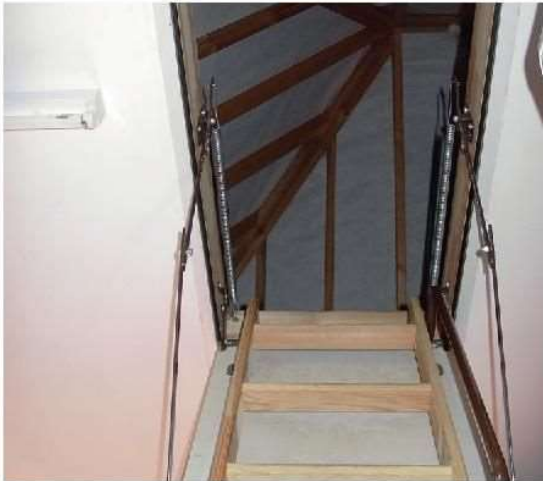
Depending upon the work activity, any space can become a confined space
